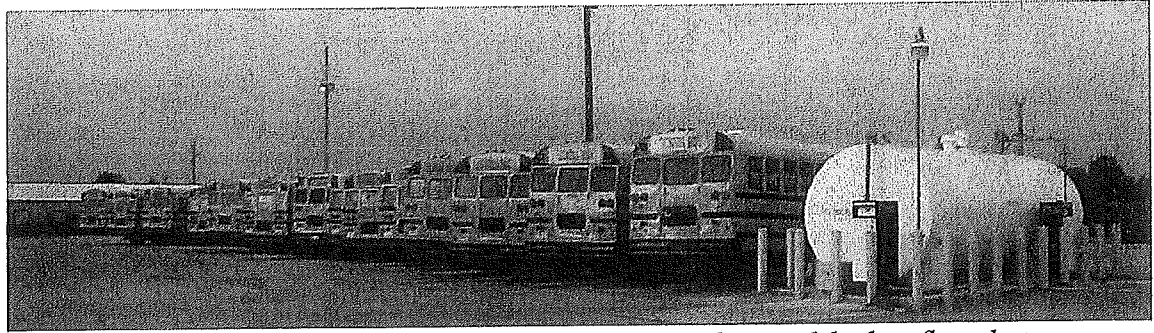
A view of the 10,000-gallon fuel tank. Also, a view of part of the bus fleet that could be used as spares if needed.
