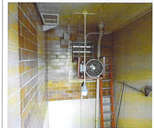
Figure 4 Unit Heater, Louver, and Ductwork Within the Wet Well Area
