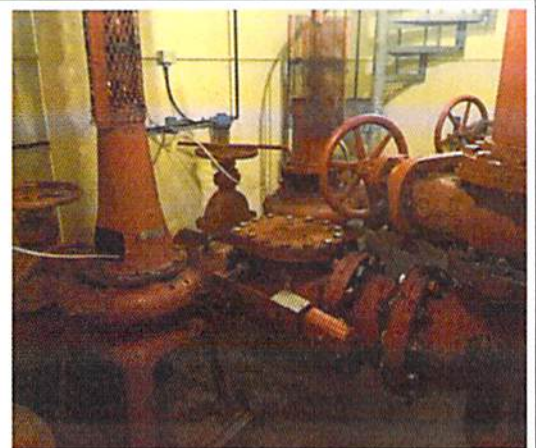
Figure 5 Existing Pump, Valves, and Piping Within the Dry Well Area
