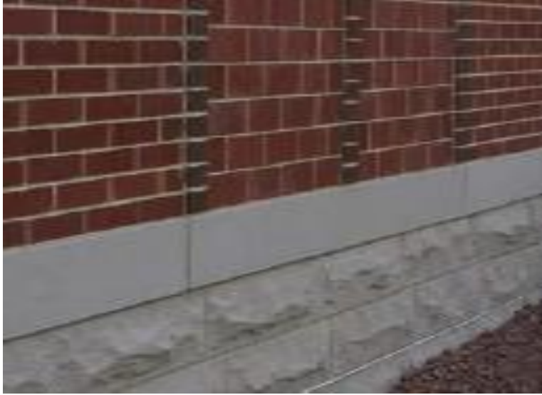
Figure C5.3via: Brick veneer is in laid in pre-cast panels. Vertical articulation features mask the joint lines.
