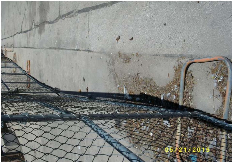
Garbage, yard waste, and other materials accumulating and left in fencing.
