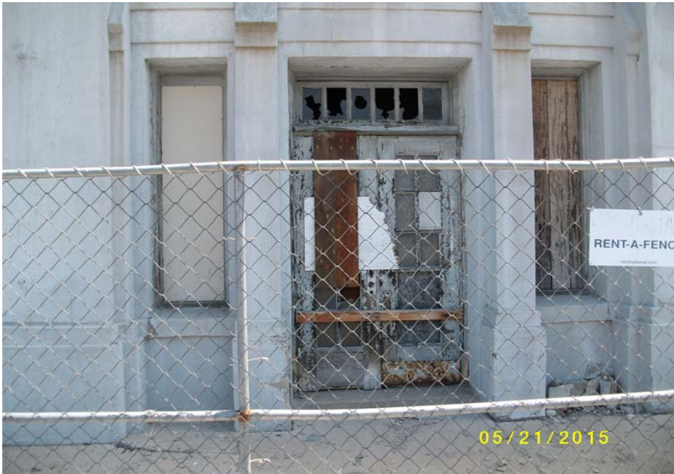
Doors damaged; not secure or weather-proof.
