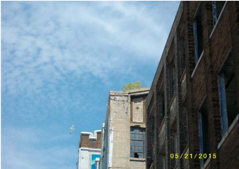
Roof conditions - trees growing on roof.
