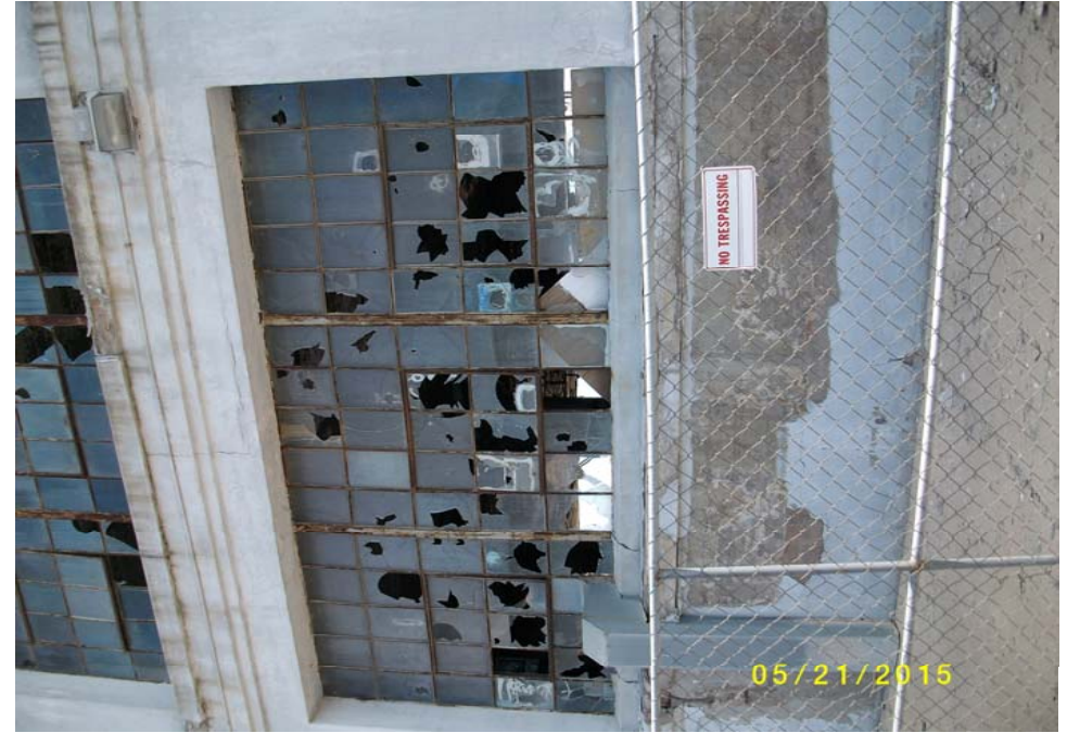
Broken glass in remaining windows.
