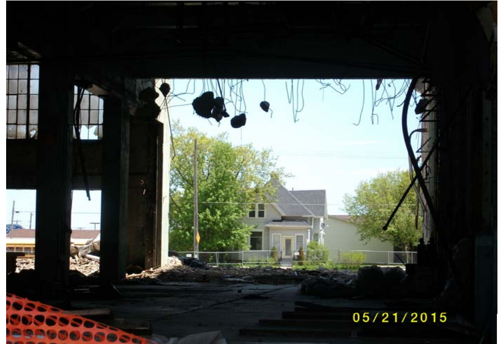
Concrete suspended above walkway.
