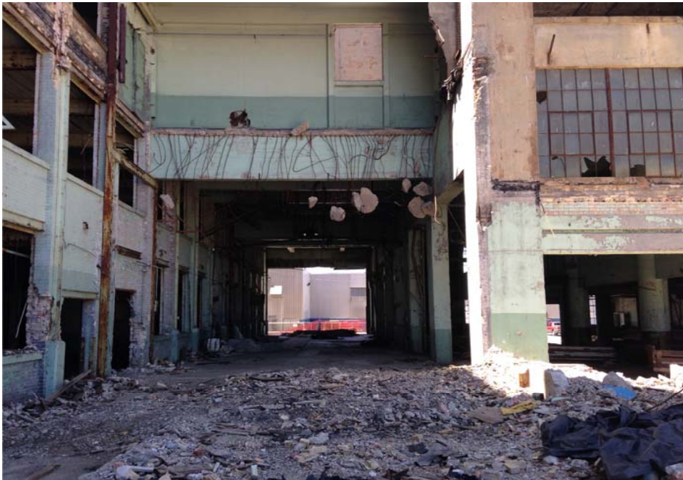
Suspended concrete left in walkway.
