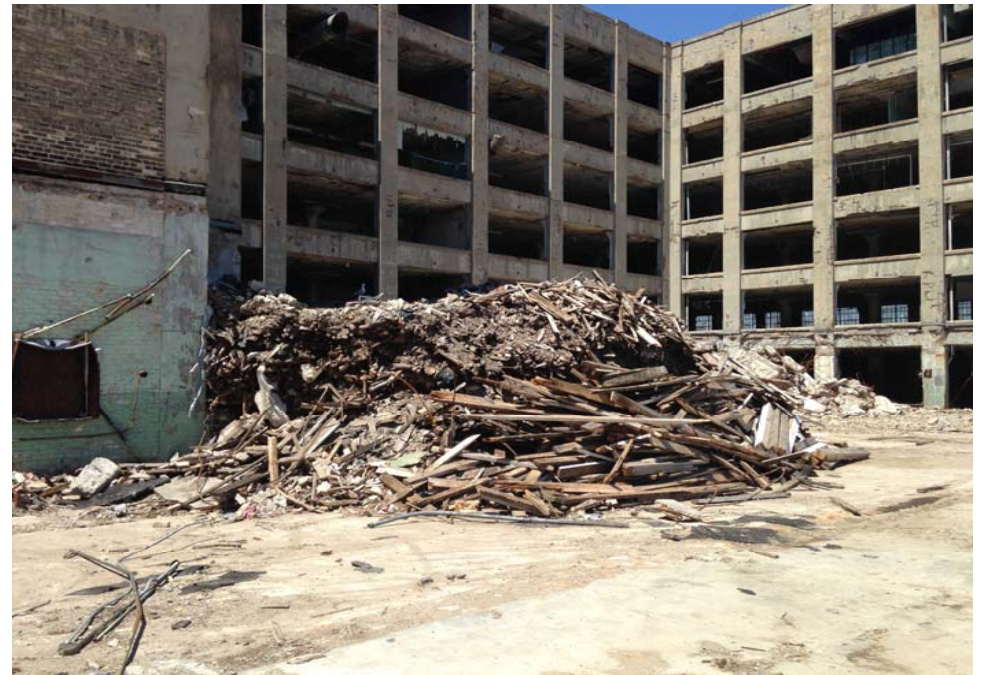
Demolition debris left on site.
