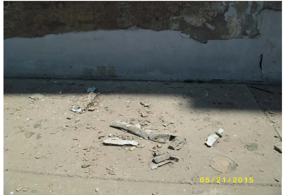
Building materials crumbling onto sidewalk.
