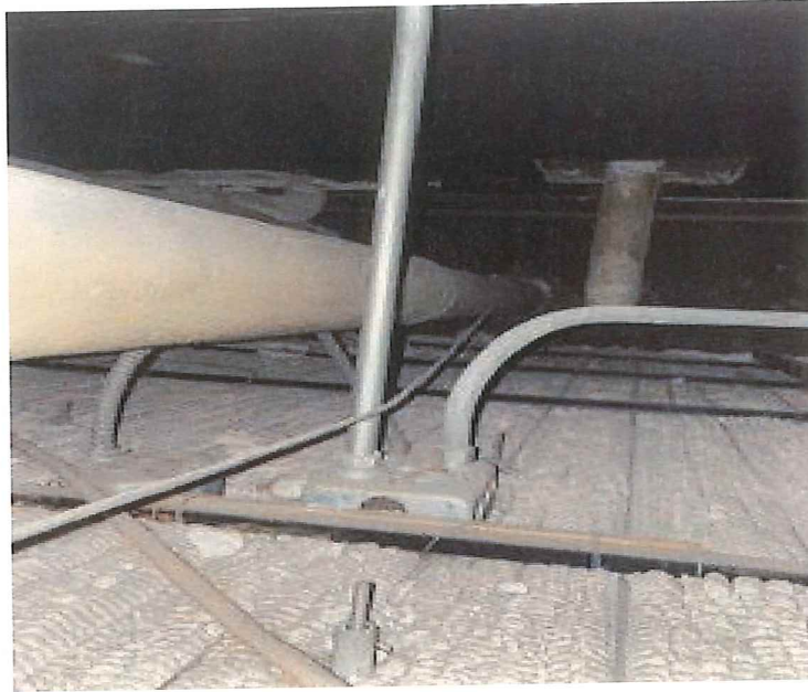
Photograph 5 – A view of the TSI on piping above ceiling outside the boiler room in the lower-level.
