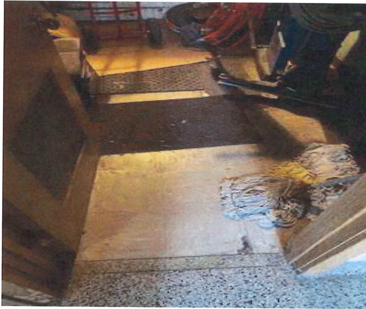
Photograph 3 – A view of the gray w/ red streaks 12"x12" floor tile and associated mastic in the lower level refrigeration/mechanical room.
