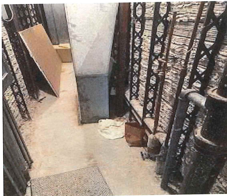
Photograph 6 – A view of the TSI on the 2 nd floor in the bathroom chase.
