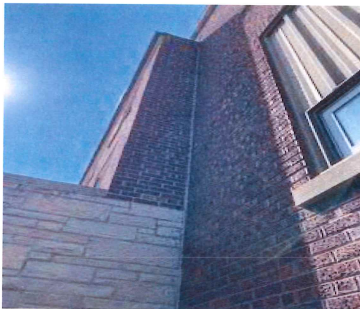
Photograph 12 – A view of the <1% gray caulking/vertical seam on the S.E. portion of the building.
