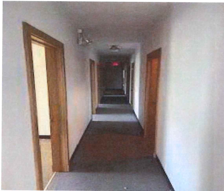
Photograph 11 – A view of a hallway on the 2 nd floor with 9”9”s beneath.
