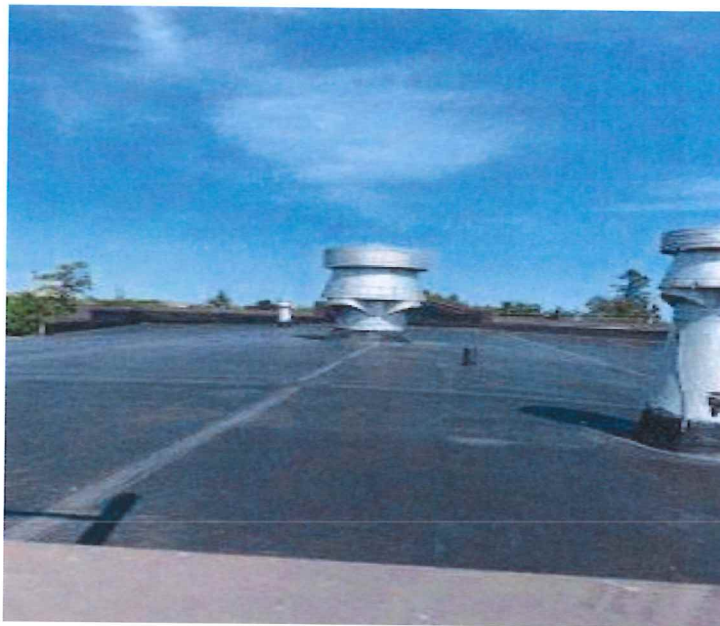
Photograph 16 – A view of the black roofing field with ACM mastic beneath.
