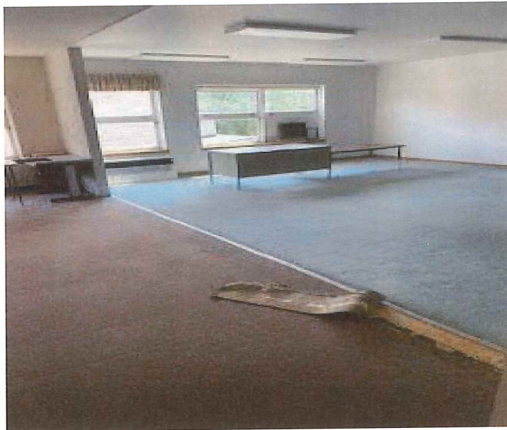
Photograph 9 – A view of the area with the black 9"x9" floor tiles in the 2 nd floor south center room.
