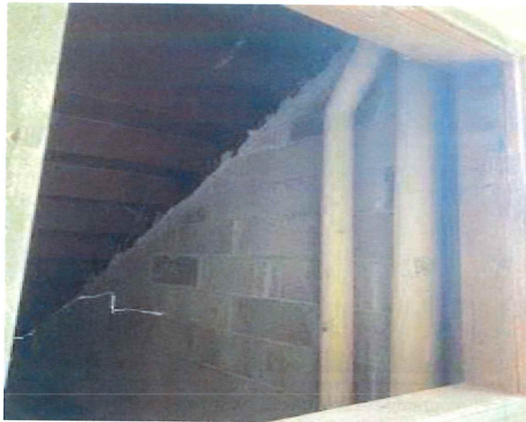
Photograph 4 – A view of the TSI on piping in the west space beneath stairs in the lower-level.
